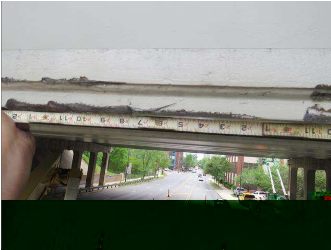
Span 2 Beam 1: Supplemental Inspection Impact Damage, The Bottom of the Beam is bent Northward for the Length of 35 Foot With the Max Distance at the Point of Impact Being 5.5 Inches. The Beam is Out of Plumb By 9 Degrees. The Point of Impact is 3 Foot 3 Inches Long and 2 Inches High and is Located in Span 2, 42 Foot 2 Inches From Bent 2. There are 3 Gouges at the Bottom of the Point of Impact: Left Gouge is 8 Inch X 2 Inch X 1/2 Inch, Center Gouge is 7 Inch X 2 Inch X 1/16 Inch, Right Gouge is 11 Inch X 2 Inch X 1/16 Inch. (PAR)
