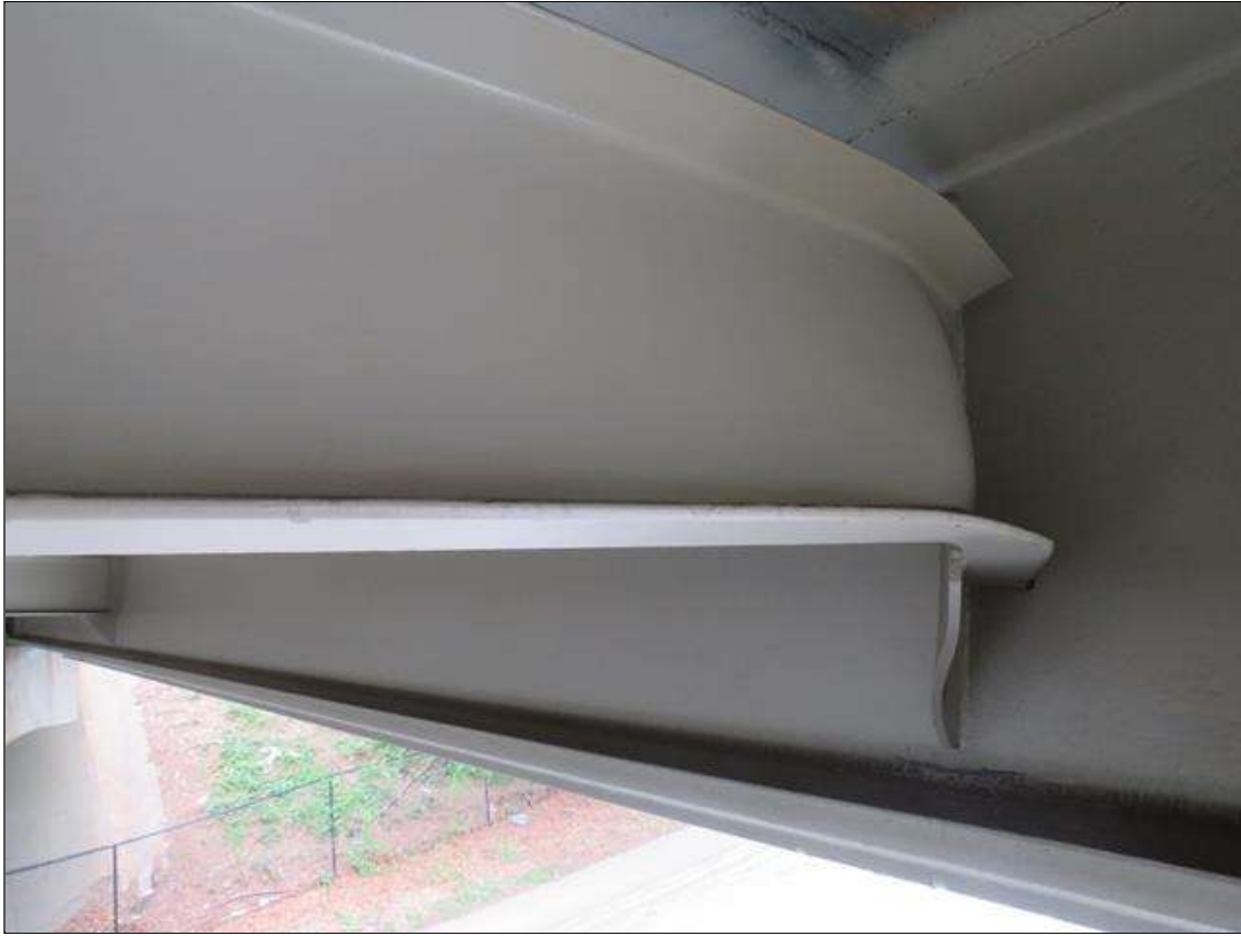
Span 2 Beam 1: Supplemental Inspection Impact Damage, Span 2 Bay 1, Diaphragm at Point of Impact Located 58 Foot From Bent 1 Has Crumpled. The Web of the Diaphragm is Distorted Up to 1 Foot. The Bay at the Point of Impact Around the Diaphragm has a Spacing of 75.5 Inches at the Top Flange and 67 Inches at the Bottom Flange. Only the Protective Coating Has Chipped and Cracked. (PAR)
