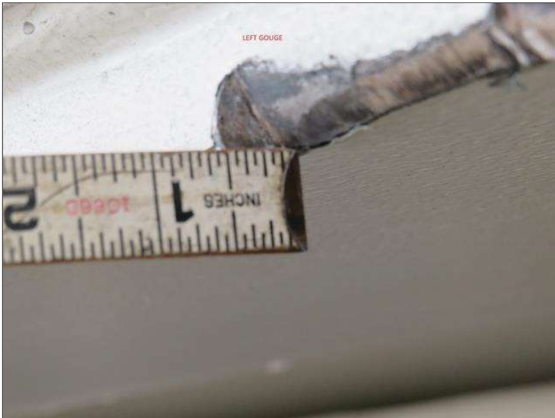
Span 2 Beam 1: Supplemental Inspection Impact Damage, The Bottom of the Beam is bent Northward for the Length of 35 Foot With the Max Distance at the Point of Impact Being 5.5 Inches. The Beam is Out of Plumb By 9 Degrees. The Point of Impact is 3 Foot 3 Inches Long and 2 Inches High and is Located in Span 2, 42 Foot 2 Inches From Bent 2. There are 3 Gouges at the Bottom of the Point of Impact: Left Gouge is 8 Inch X 2 Inch X 1/2 Inch, Center Gouge is 7 Inch X 2 Inch X 1/16 Inch, Right Gouge is 11 Inch X 2 Inch X 1/16 Inch. (PAR)
