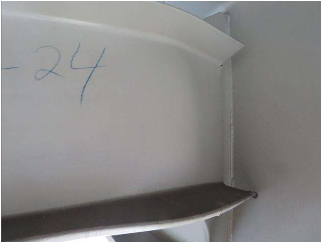
Span 2 Beam 1: Supplemental Inspection Impact Damage, Span 2 Bay 1, Diaphragm at Point of Impact Located 58 Foot From Bent 1 Has Crumpled. The Web of the Diaphragm is Distorted Up to 1 Foot. The Bay at the Point of Impact Around the Diaphragm has a Spacing of 75.5 Inches at the Top Flange and 67 Inches at the Bottom Flange. Only the Protective Coating Has Chipped and Cracked. (PAR)
